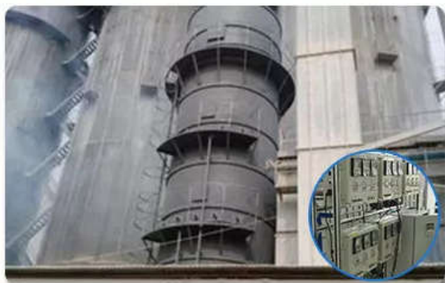
— Acid alkali waste tower —
