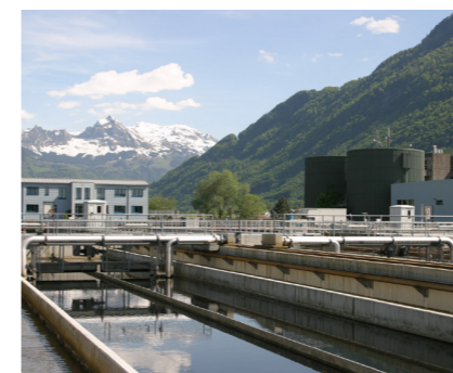
Water and wastewater treatment
