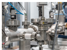
Industrial water treatment
